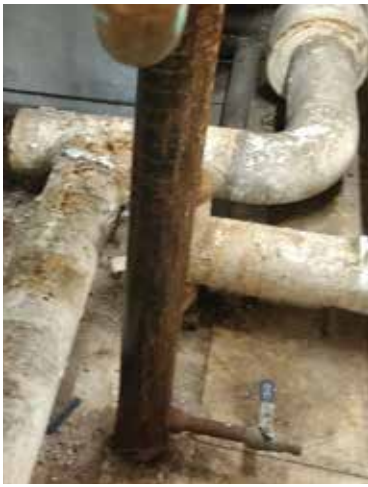
Heating Plumbing Pipes
