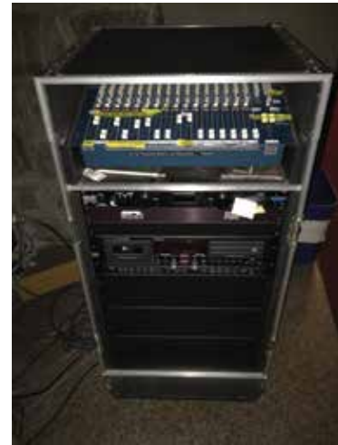
Nave Audio System
