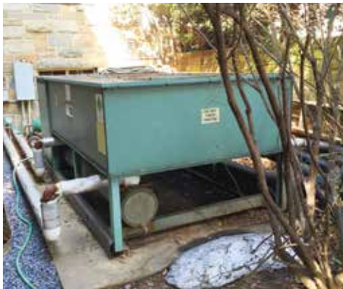
1950s HVAC System
