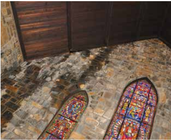
Nave West Wall Water Damage
