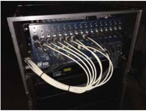
Nave Audio System
