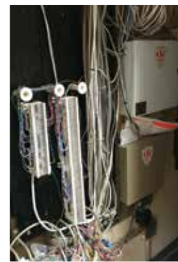
Outdated Wiring, Phone Circuitry and Breaker Panels
